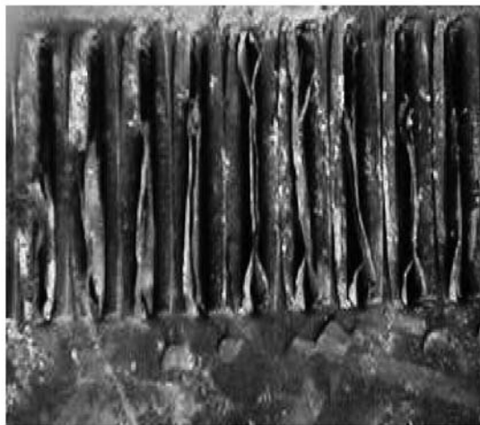
Example 2: PPL separated from base metal due to sulphuric acid attack
